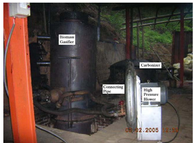
Fig. 12. Integration of the bamboo carbonization kiln and biomass gasifier.
